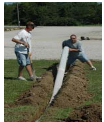
Greg Misel and Aaron Arthur install line to bring water off of field #1.
