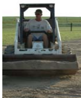
Greg Misel in bobcat delivers sand to the tiles to cover the drainage system.
